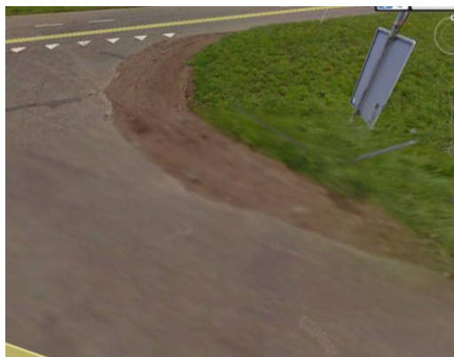
Bermschade in bocht (bron: Google Earth)
